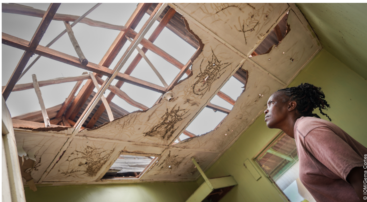
A resident explains how her roof was torn off by Hurricane Beryl, Jamaica 2024
