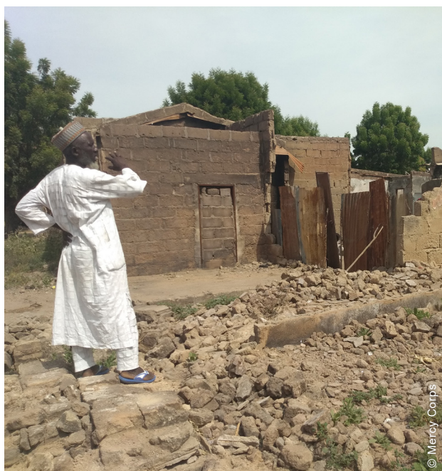
A completely damaged shelter in Bama Local Government Area, Borno State.
