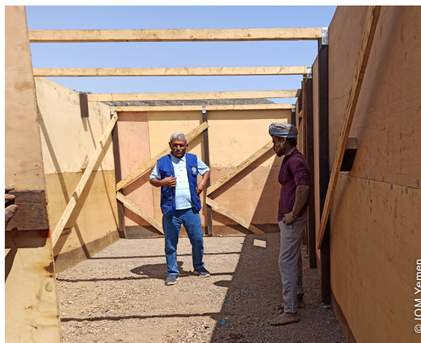
Organization provided technical assistance and conducted training sessions on shelter construction and maintenance for the targeted households.
