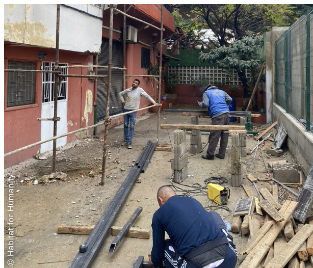
Construction work on a building facade as part of the urban recovery project.
