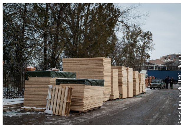
Reconstruction work began as soon as some areas were liberated from the presence of Russian troops.
