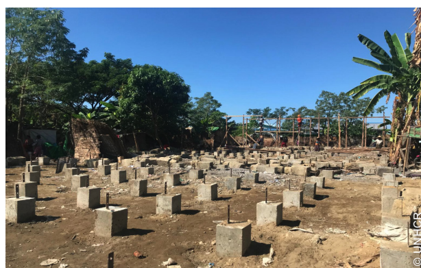
The reconstruction work incorporated pre-cast footings for extending the lifespan of the timber frames, while improving the anchorage of the building to the ground.
