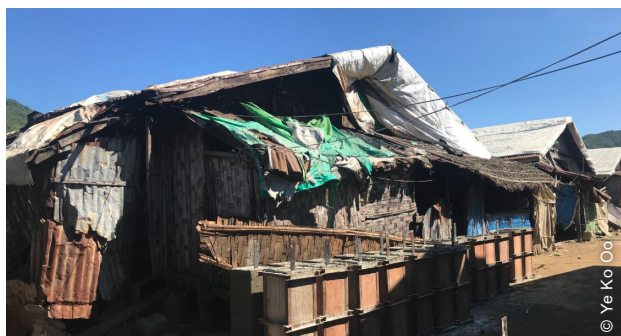
Damaged shelters in Sittwe Township camp, March 2022.
