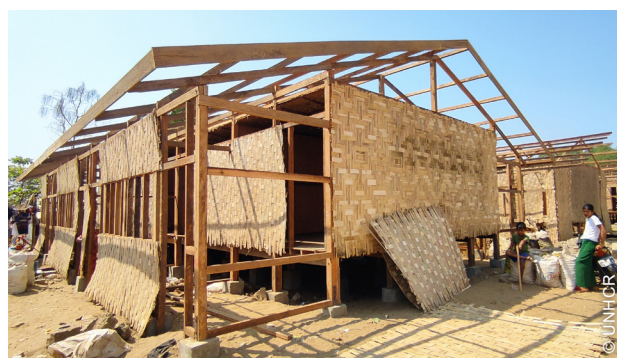
The reconstruction works included the replacement of the timber frame and bamboo cladding elements of the longhouse.
