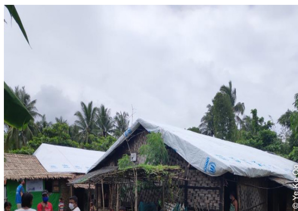
'Mega-tarps' used to cover shelters not marked for reconstruction ahead of rainy season. the project, June 2022.
