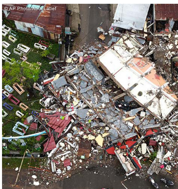
An aerial view of a damaged building following the earthquake in Mamuju, West Sulawesi.
