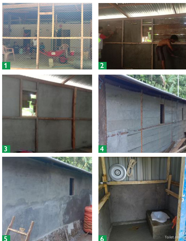
1: Construction training; 2: First formwork; 3: Inner plastering; 4: Outer plastering; 5: Outer plastering completed; 06: View of a completed room.
