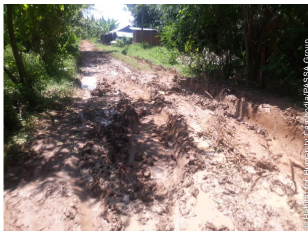
Damaged roads after the impact of flooding. The community projects implemented included the renovation of roads, amongst others.
