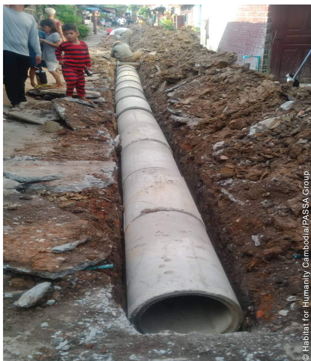
The project provided grant support to the groups to renovate the community's water drainage system.
