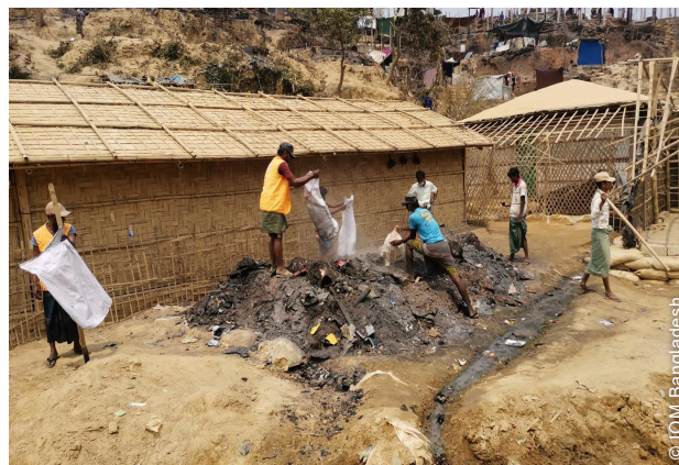
Debris removal started immediately in the initial phase of the response in both the fire incidents, involving many community volunteers and laborers.
