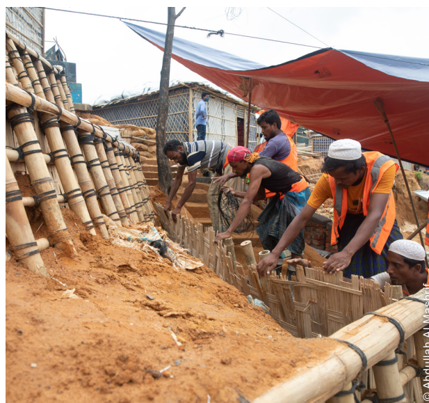
Site development work of reconstruction of bamboo slope stabilisation and access carried out by people engaged in Cash for Work, February 2022.
