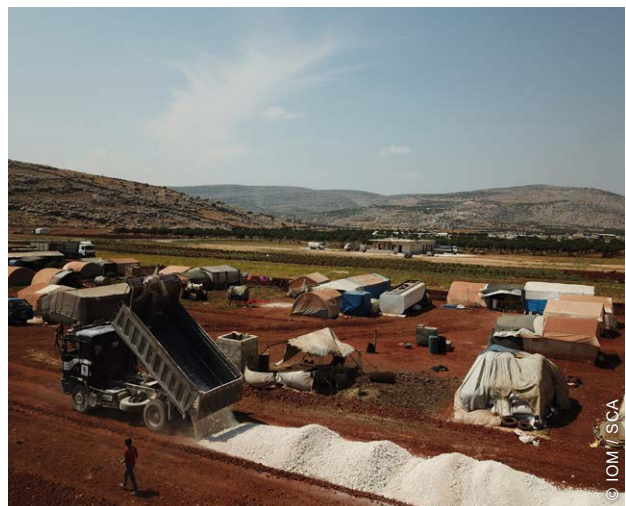
Implementing Partners coordinated with site residents to try to minimize disturbance during site works.
