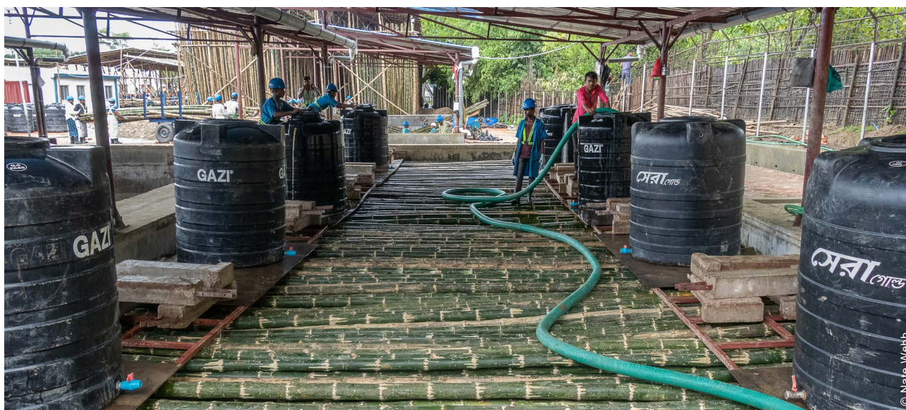
The orthoboric solution used for the treatment of bamboo was selected for its ease in processing and its non-toxic nature.
