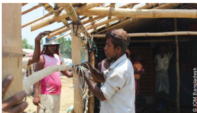
By involving refugees throughout the implementation, the project helped generating a sense of ownership over the shelters and their surrounding environment.
