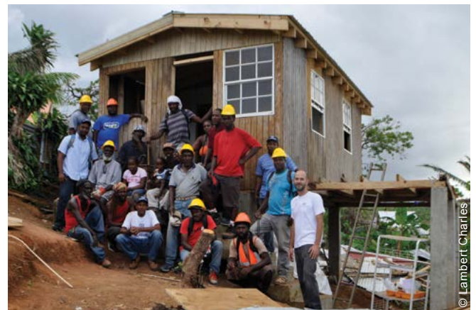
For vulnerable households with a completely destroyed house, core houses were built according to a locally approved studio design. Due to its cost, targets had to be adjusted.
