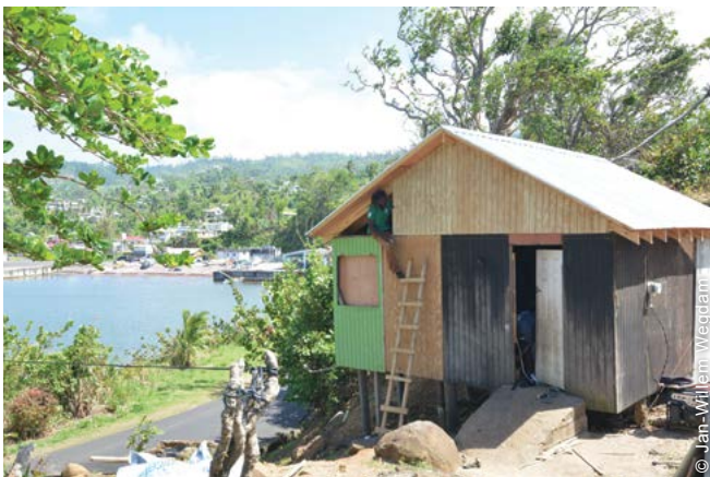
The project repaired 670 roofs in compliance with an improved building code after the hurricane.
