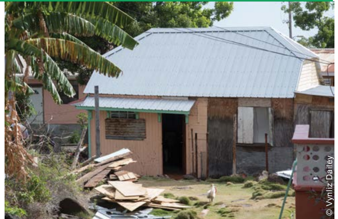
Even though roofs were repaired to code, structural improvements were not considered, nor were water, sanitation and livelihood components.
