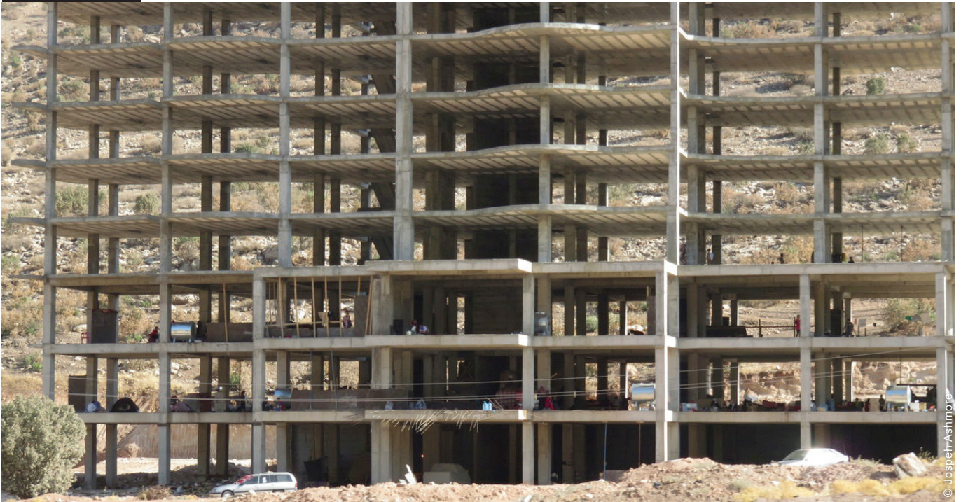
Unfinished buildings were occupied by some people. Where agreements were possible with landowners, repairs, light or durable upgrades were made. In some cases, frame tents or sealing-off kits were provided.
