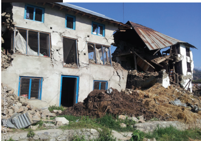
Many constructions affected by the earthquake were masonry buildings. The project provided materials to make urgent repairs to damaged homes, or build temporary shelters.
