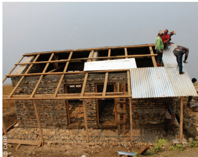
Houses were repaired also using the materials provided by humanitarian organizations, such as CGI sheets and timber.
