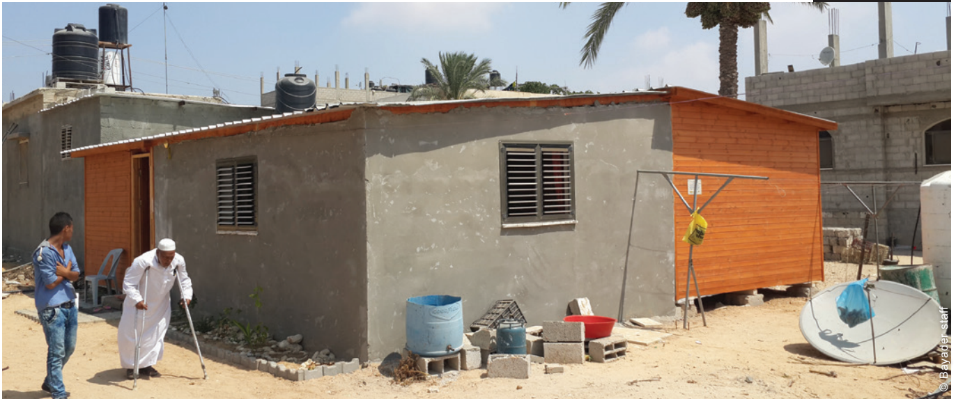
Some people were able to extend the shelters, by closing the open sides of the veranda.
