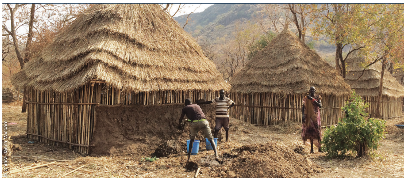
Refugees plastered the walls of the shelters with mud, made from soil sourced by the refugees themselves, in areas agreed with authorities and host communities.
