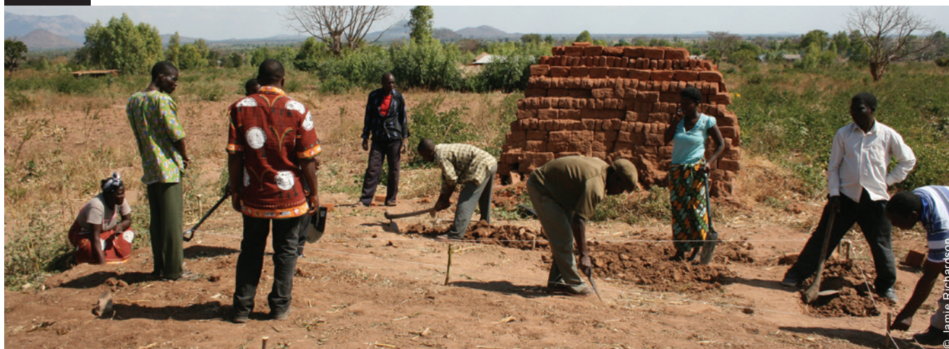
People were given technical trainings and built model houses as part of the project. Here they are working on setting out the foundations of a model house..
