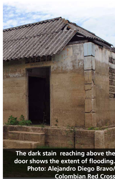
The layout of the old village. The site was severely flooded on separate occasions over many years. Photo: Alejandro Diego Bravo/Colombian Red Cross
