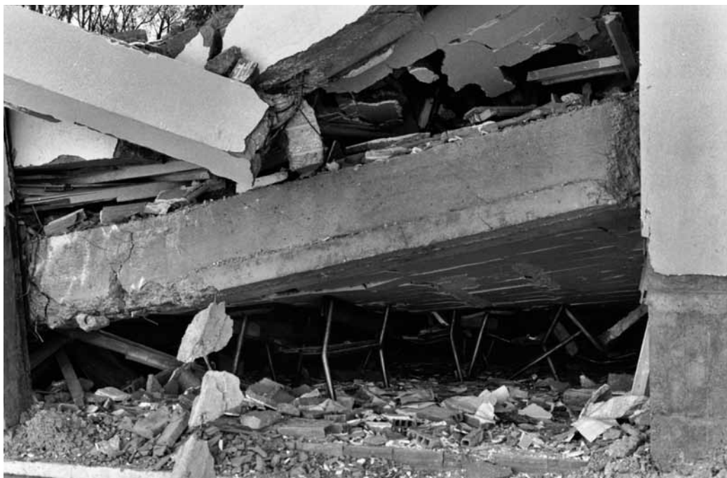
Collapsed school in El Asnam, Algeria, 1980. Act of God or Criminal Negligence? Photo: Giles Whitcombe
