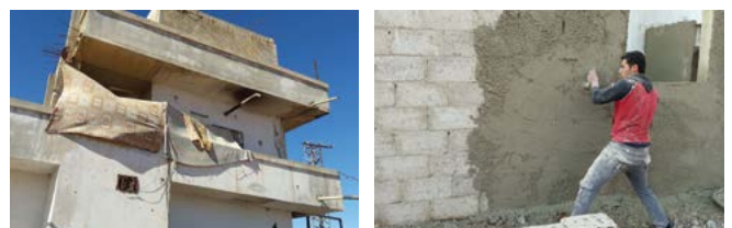
The legal team assessed each building and confirmed if works could be conducted. While this ensured HLP issues were mitigated, it also meant that some households had to be left without assistance.
