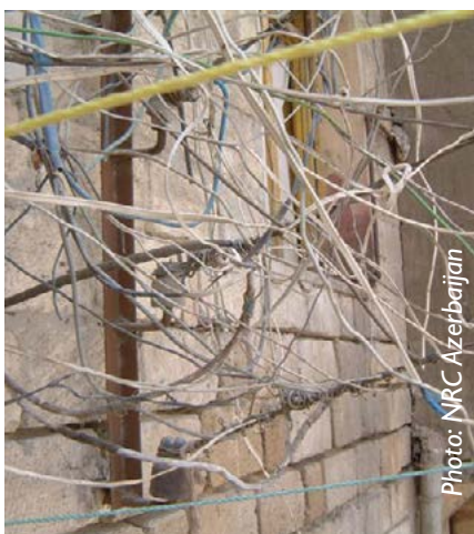
Wiring before upgrade
