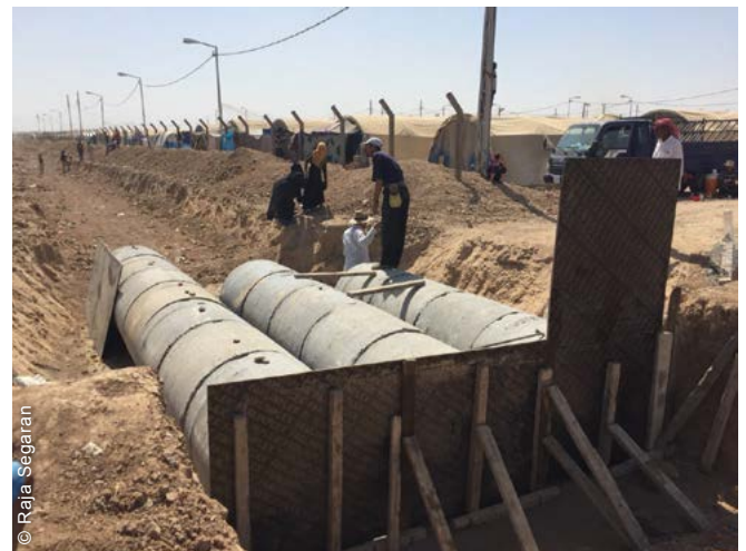
One site was vulnerable to heavy rains and suffered minor flooding during winter. In 2018, storm-water drainage channels and culverts were upgraded.
