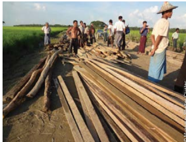
© Myanmar Shelter Cluster Construction materials were supplied by the government to rebuild the houses of IDPs affected by the violence (Thi Kyar IDP Camp, Mrauk-U Township).
