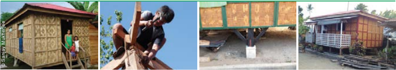
Safer building practices were promoted, such as strapping of roof structures, bracing and proper detailing of the foundations (raised and made of reinforced concrete).
