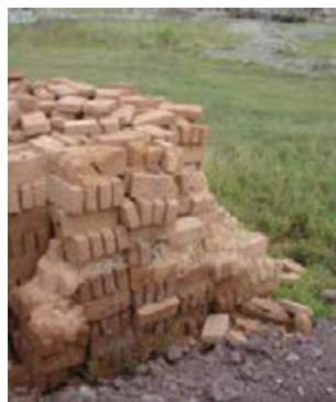
Obtaining good quality building materials remained problematic. These bricks decayed rapidly in the rain.
