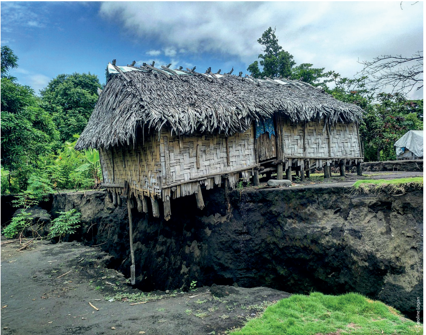
Ambrym Earthquake and volcano damage in January 2019.
